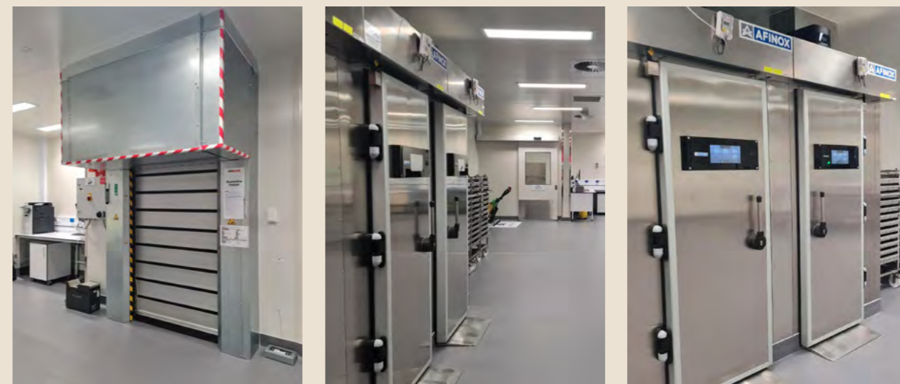
Highbrook features a quarantine freezer (left) and four blast freezers (right), which will ultimately become eight, enabling 672 units of plasma to be frozen at a time. Currently, the Epsom-based operation has just two freezers which blast-freeze 84 plasma units within an eight-hour freezing cycle.
